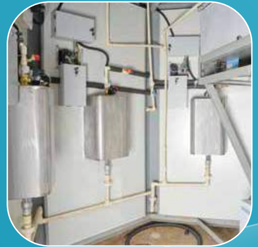
Inside the plant
